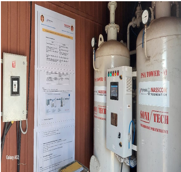
The oxygen generation plant is a 2 PSA Tower/ sodium Zeolite Molecular Sieve with 10 year life span & a 6 stage filtration process.
